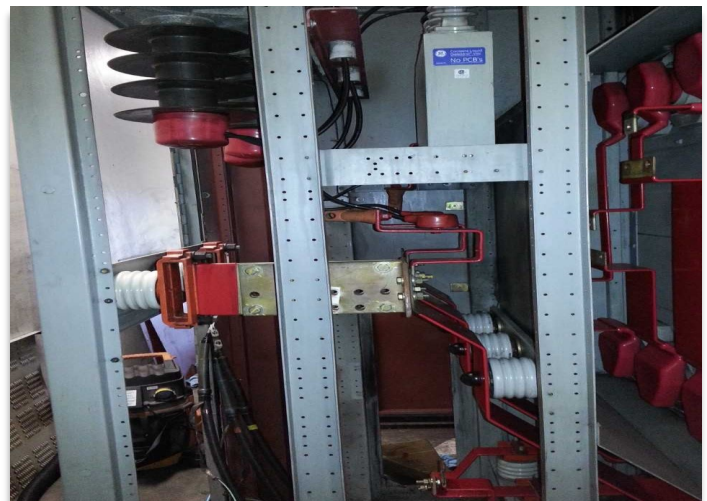
High Voltage Switchgear Motor Control Center at the South Campus Chiller Plant
