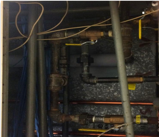
Replacement of Non-Functional Heating Hot Water Valves at the Center for Visual Arts
