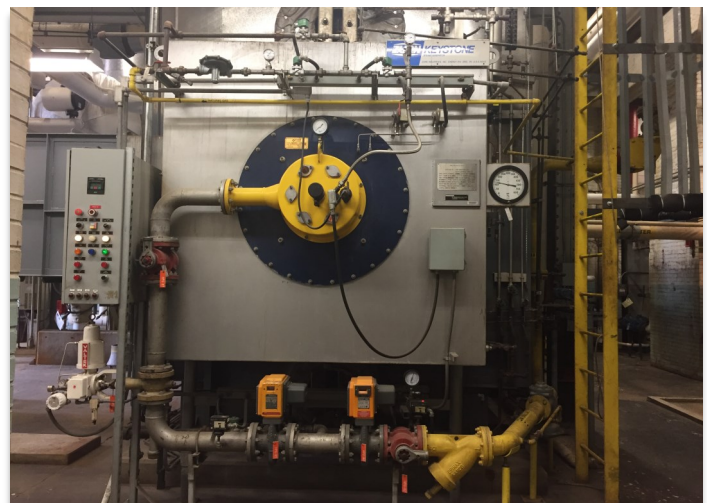
Boiler#8 at University Heating Plant
